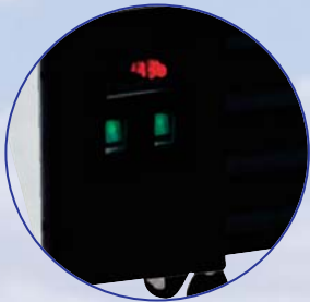
Digital Control Panel
